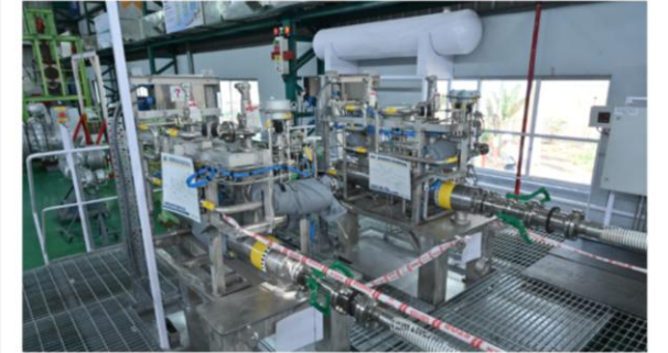
To train seafarers, Anglo-Eastern has an LNG/ammonia bunkering station skid at its academy in Karjat, Mumbai (source: Anglo-Eastern)
